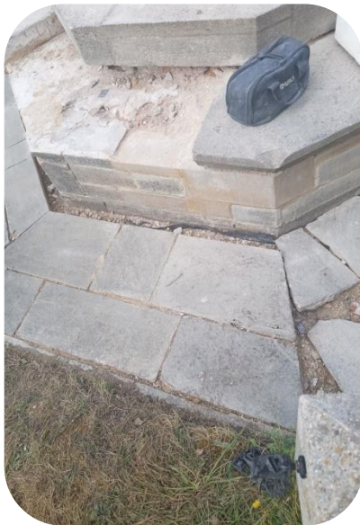
20/08/2024 - The old damaged coping stone has been removed and awaiting the new coping stone to be fitted.
