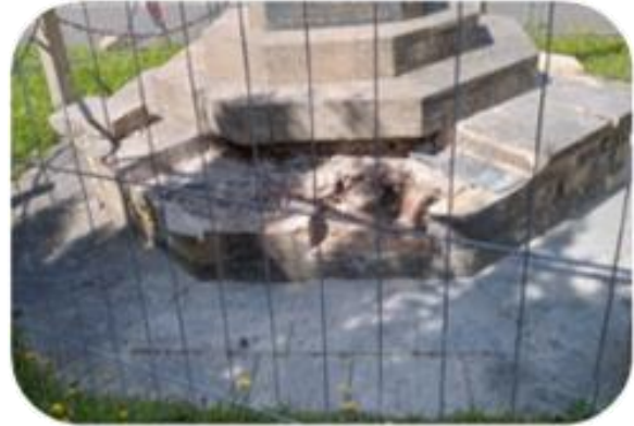
18/07/2024 - The inside of the structure is drying out.
