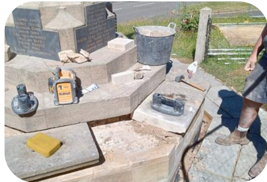
16/08/2024 - Coping stones being carefully replaced using a suction tool to accurately place the coping stone in the correct position.
