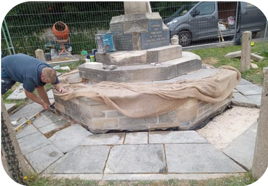
14/08/2024 - Levelling of the ground using a spirit level whilst work continues in the contractors work shop to cut the replacement stones to size.
