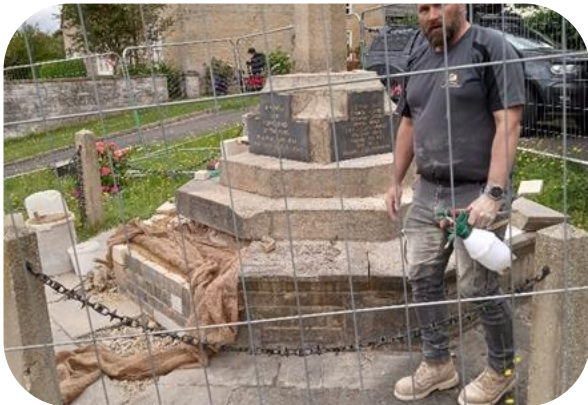
25/07/2024 - Specialist cleaning of the existing stones before the new stones are laid.
