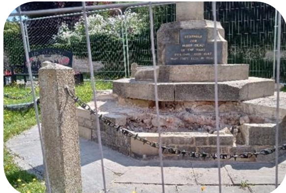
23/07/2024 - The inside of the structure can be clearly seen having dried out.
