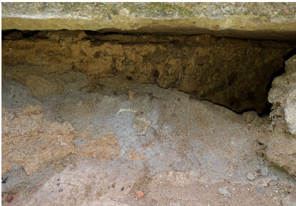
Grey Hard Cement used to bed coping stone in a previous phase of repairs
