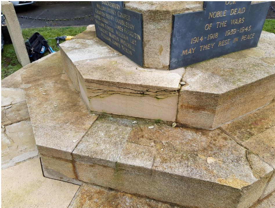
Failed Ancaster Stone
