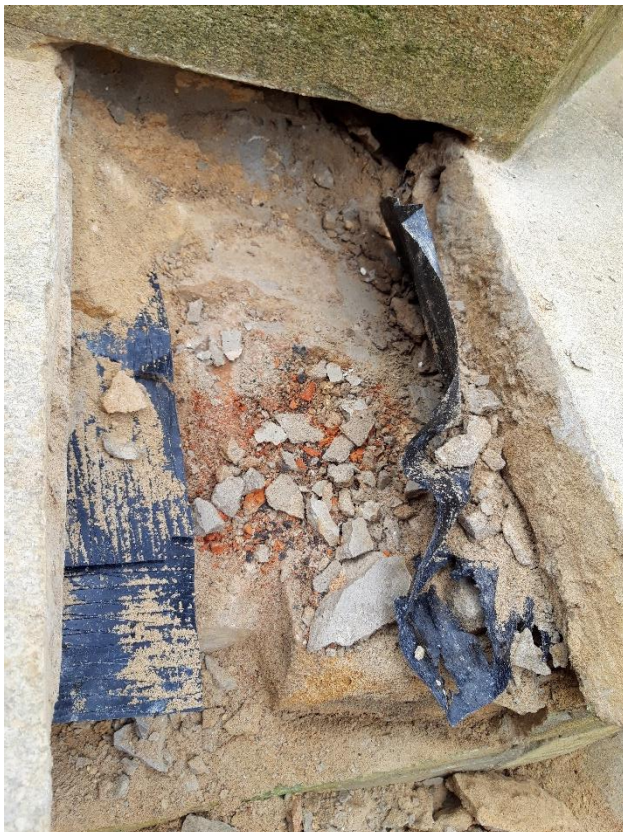
Damp proof course following removal of the coping
