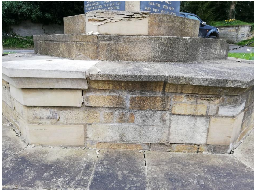
Fig. 2: The Northwest plinth elevation (side B on plans) with failing Ancaster stone to step 3 of the base plinth.
