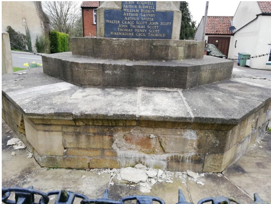
Fig. 7: The East side as found at a site visit over a year after the investigative section: the plastic repairs to the stone have already fallen off which is an indication of the high water retention inside the plinth
