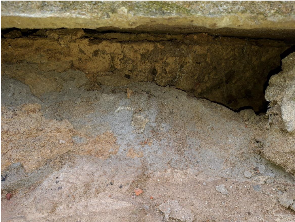
Fig. 5: The grey hard cement used to bed coping stone in a previous phase of repairs needs to be removed.
